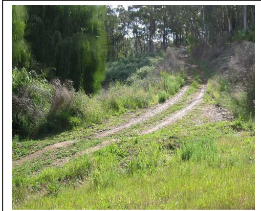
This well constructed track has been shaped with a wide, grassed drain (right of track) to transport water, and a cross drain (foreground) to carry water safely over the track. It has been surfaced with rubble and is well compacted
