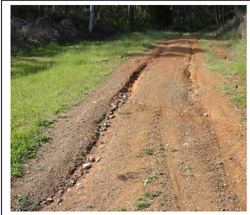
Without a good drainage system, tracks will erode, like this one.
